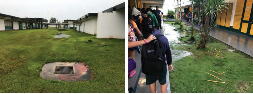
Figure 10: These grass swales do not convey water to the drain inlet or away from the sidewalks and need to be re-constructed.
