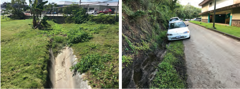
Figure 8: Mud, grass and weeds in concrete and grass swales block the flow of stormwater, causing poor drainage.
